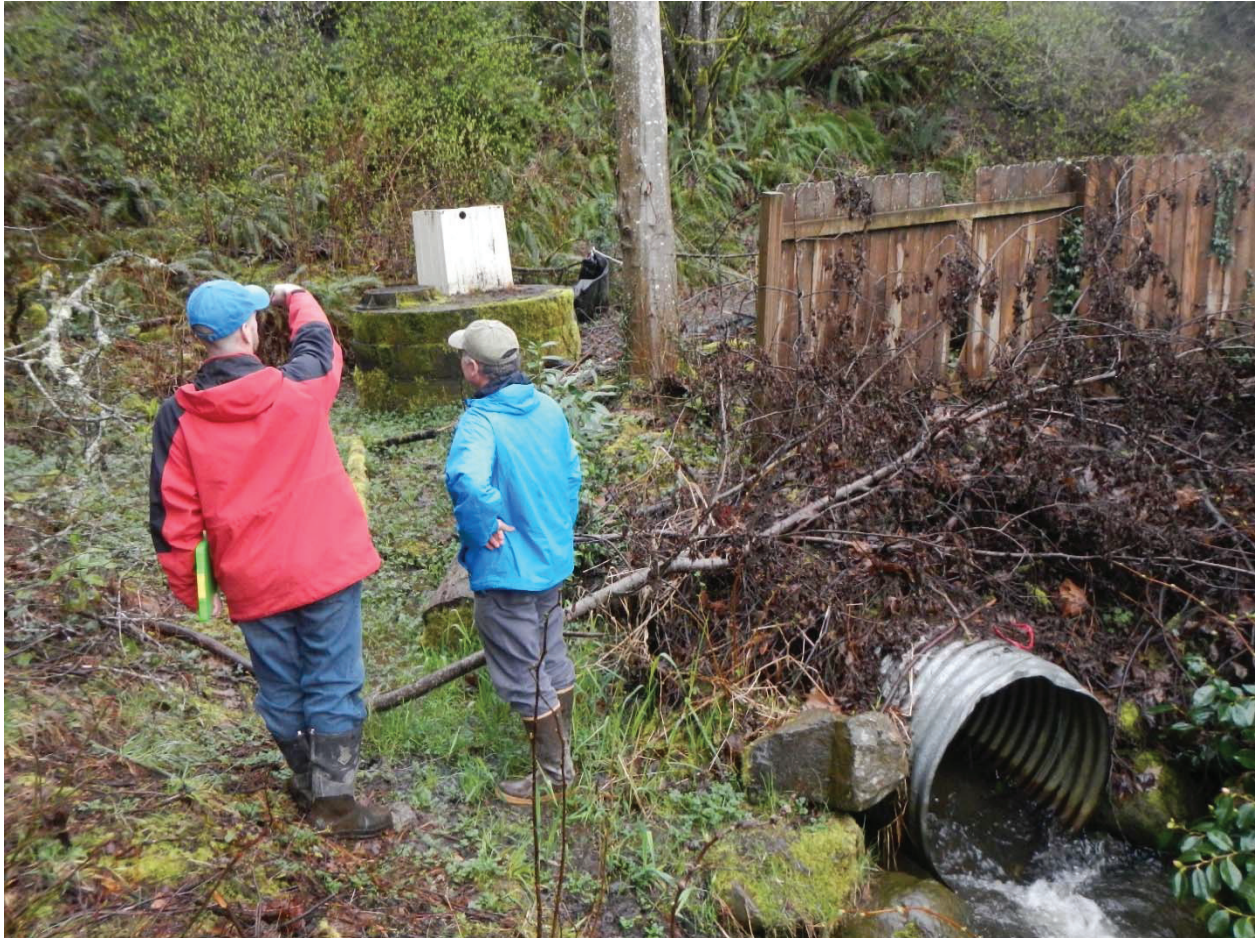
Photo 1: 36-inch CMP outfall to flood-prone open channel reach downstream of Colchester Drive.
