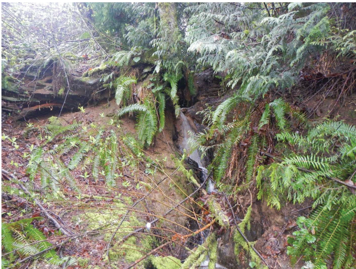
Photo 6: Right bank drainage at intersection of Colchester Drive road fill and Duncan Creek valley wall. Drainage likely initiates from both Colchester Drive to south of Duncan Creek and Puget Drive to southwest.
