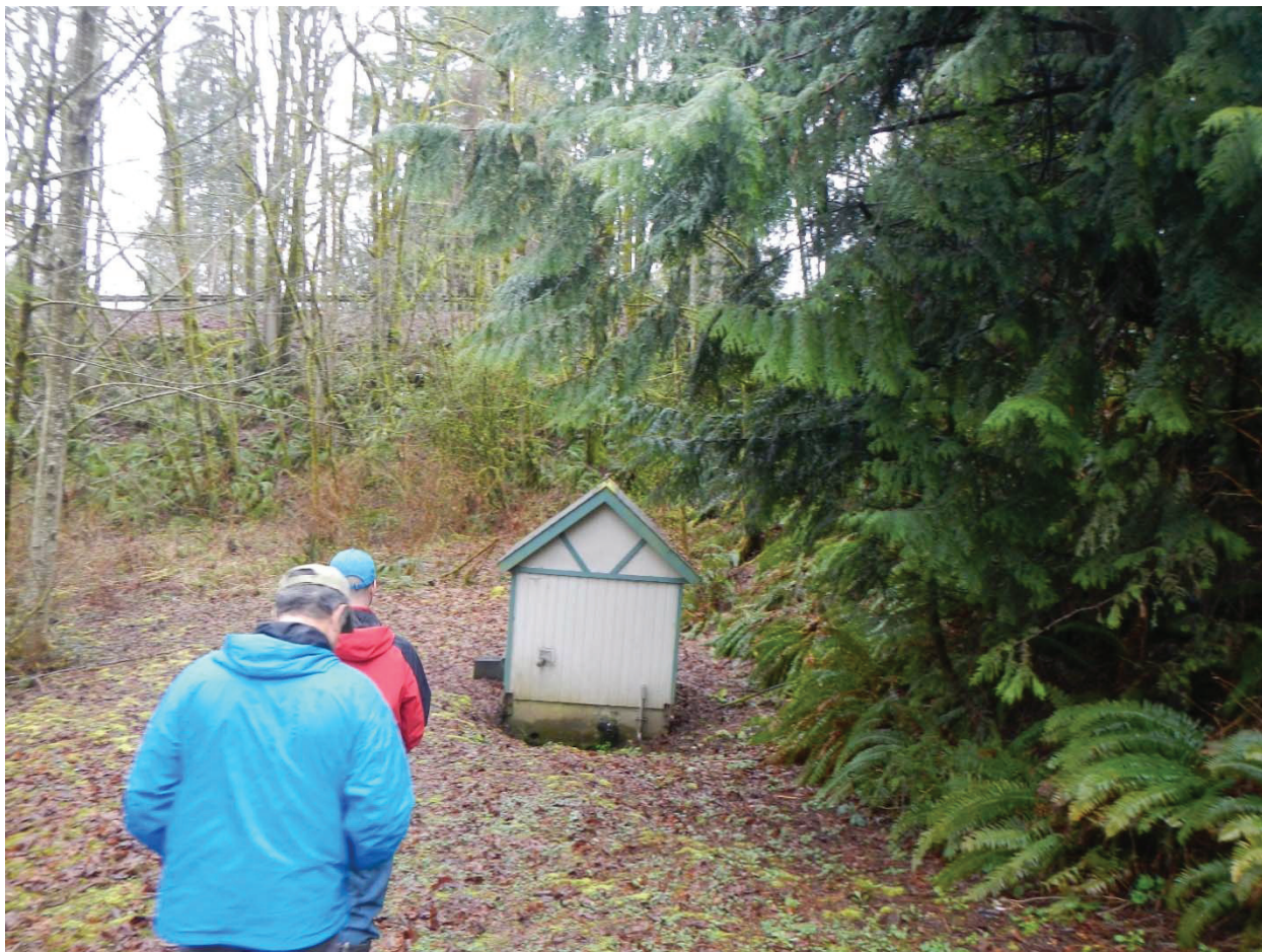
Photo 7: Water District infrastructure on right bank upstream of Colchester Drive road fill.
