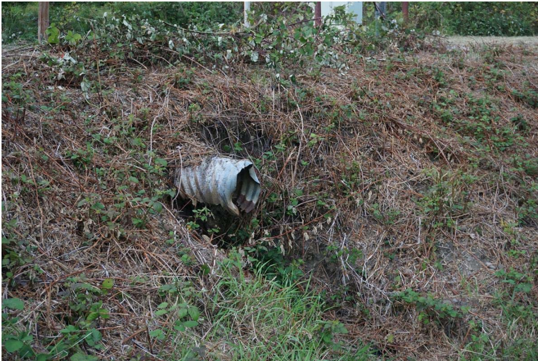
Water drips from a culvert in a drainage ditch along Kresky Ave.
