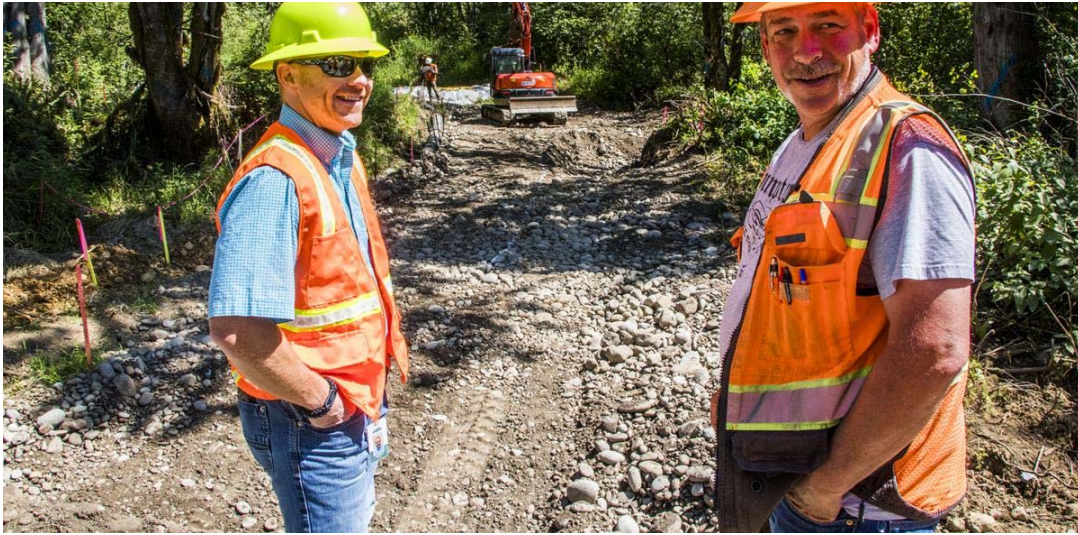
Public Works director Josh Metcalf, left, and Bridge Inspector Joe Byers, right, look over progress at the Pigeon Springs fish barrier removal project Tuesday afternoon. Jared Wenzelburger / jwenzelburger@chronline.com
