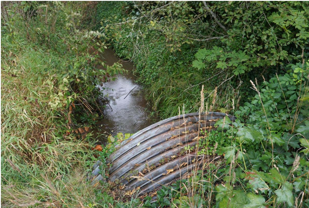
Scammon Creek flows beyond a culvert under Graf Road. The metal pipe, which obstructs the passage of salmon, is one of many Lewis County is looking to replace in the coming years.
