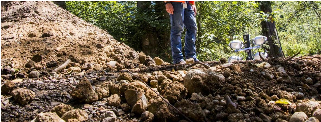
Public Works director Josh Metcalf looks on at the progress at the Pigeon Springs fish barrier removal project Tuesday afternoon.
