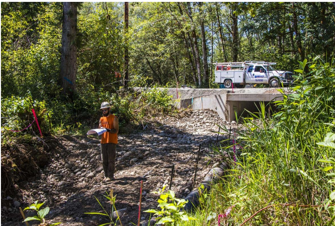
Crews lay fish rock during the Middle Fork Newaukum fish barrier removal project Tuesday afternoon.
