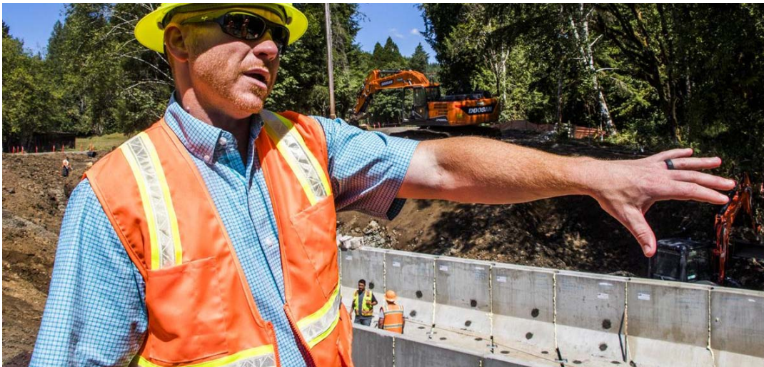
Public Works director Josh Metcalf talks about what crews are doing at the Pigeon Springs fish barrier removal project Tuesday afternoon.
