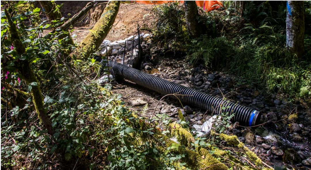
The Middle Fork Newaukum fish barrier removal project bypass pipe lets water flow while crews work on putting down fish rocks in the area where the water normally flows, Tuesday afternoon.
