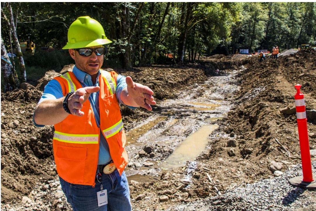
Public Works Director Josh Metcalf motions to an area at the Pigeon Springs fish barrier removal project Tuesday afternoon.
